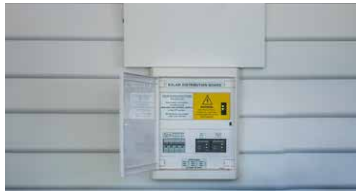
The electrification upgrade included an Induction Cooktop & Solar Distribution Board
